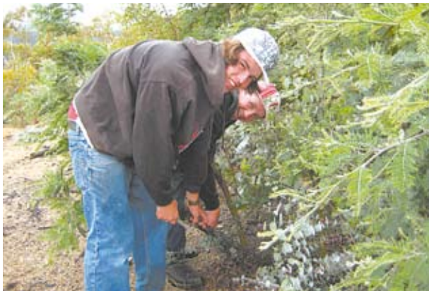
Year 10 work experience students Dan Kroenert (front) and Joshua Heath from St. Patrick's Parish School in Cooma removing redundant tree guards and stakes as part of the Waste Point Tip rehabilitation project (photo by Dave Woods).
